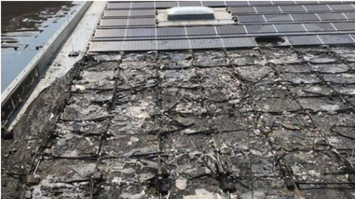
Figure 11 Damage on the roof of Gazelle (source: www.omroepgelderland.nl )
