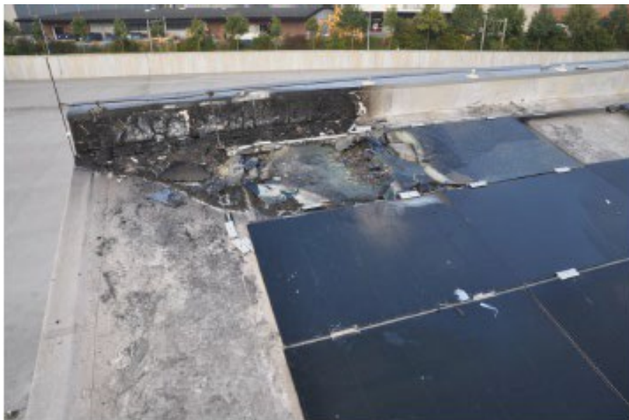
Figure 15 Fire damage limited to a few panels and a small part of the roof.
