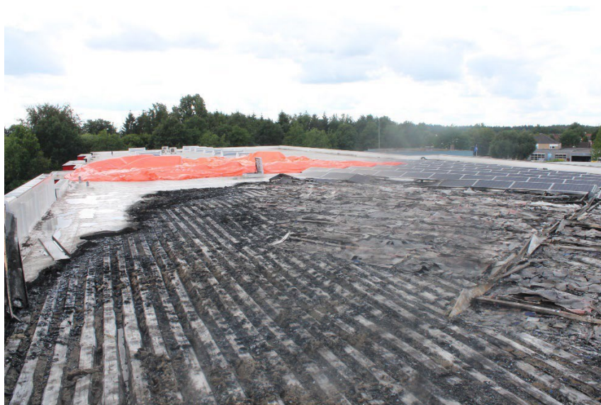
Figure 4 The fire has been stopped before the fire separation (at the location of the tarpaulin on the roof) (source: Fire brigade Twente)
