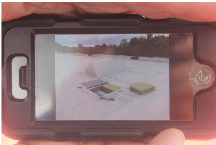
Figure 5 The roof is interrupted at the fire-resistant partitions with rock wool, but not covered with a layer of concrete tiles (source: Fire Department Twente)
