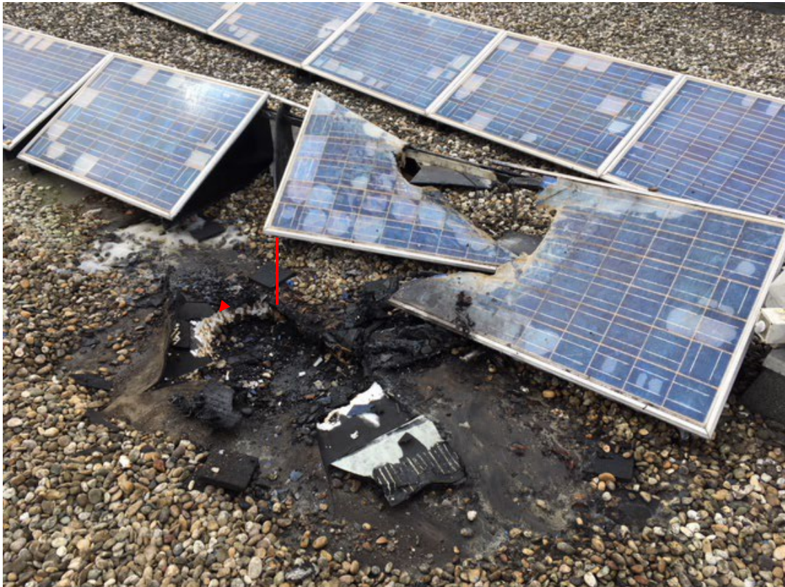
Figure 8 Damage to solar panels and roof. Melted EPS is visible in the red arrow. Characteristic "caramelised drops" (source: Municipality of Opmeer)
