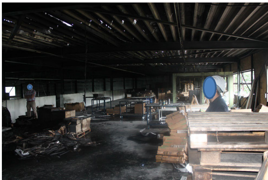
Figure 6 Secondary fire in the building caused by burning falling material (source: Fire brigade Twente)
