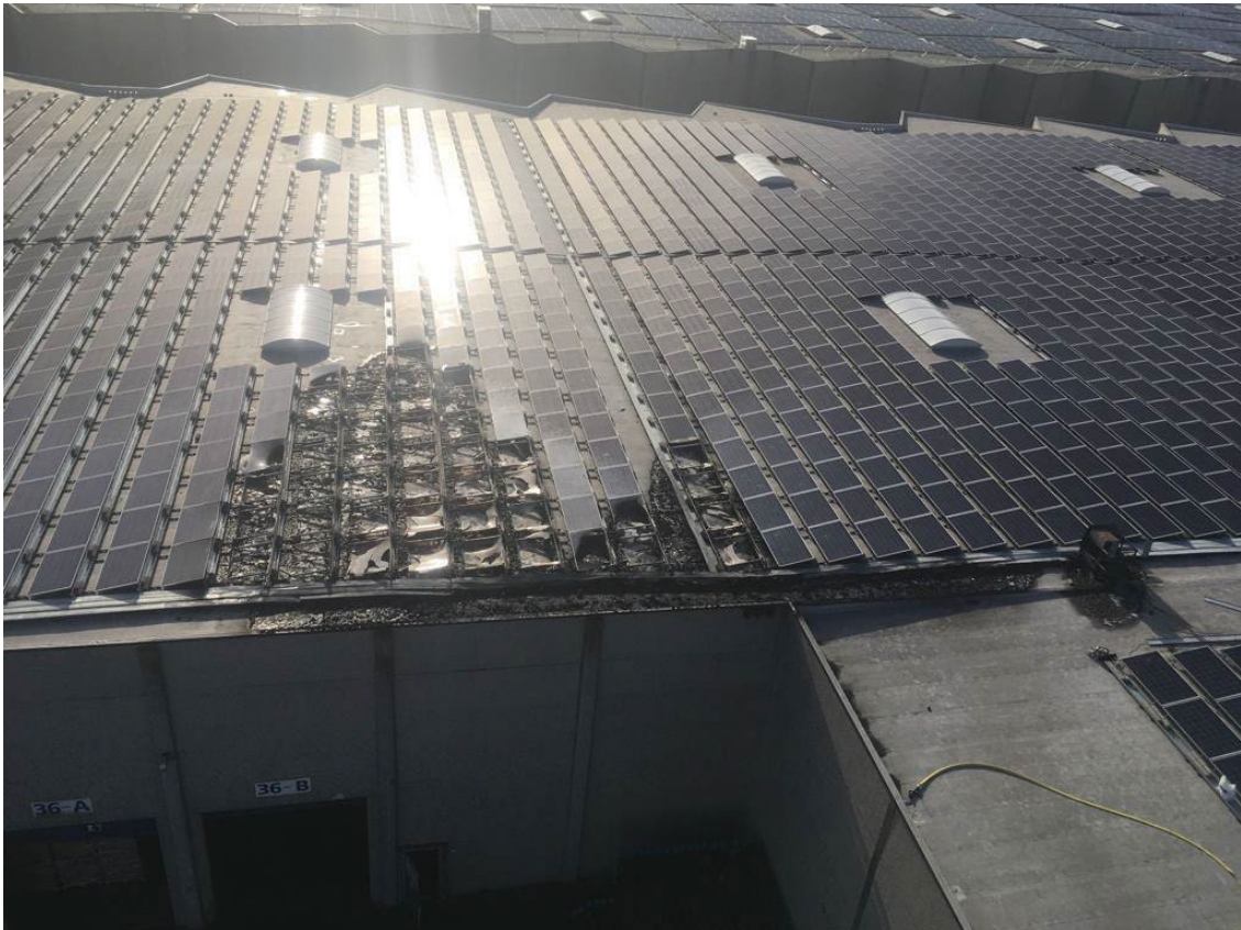
Figure 9 Damage on the roof of the storage hall (source: Amsterdam-Amstelland Fire Service)
