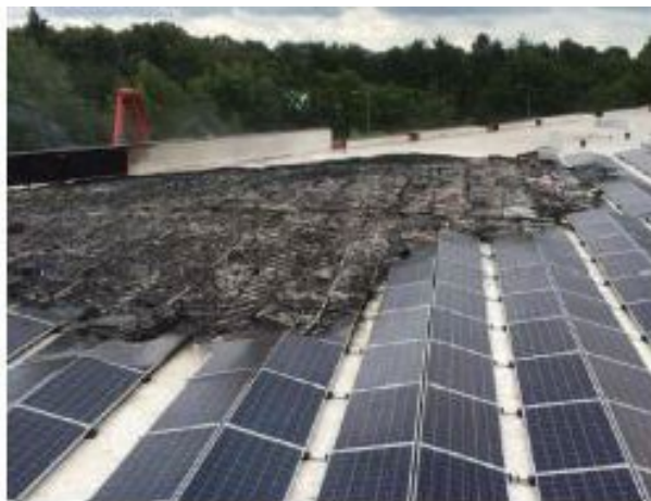
Figure 2 Overview of damage on the roof (source: unknown)
