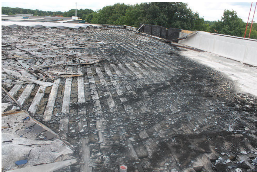
Figure 3 Damage to the roof (source: Fire brigade Twente)
