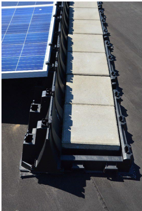
Figure 14 Plastic support structure
