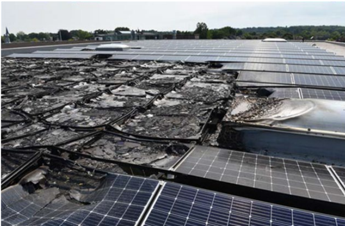
Figure 12 Damage on roof of Gazelle, where the fire reached a skylight (source: unknown).
