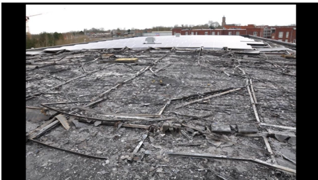
Figure 17 Damage to the PV plant and roof (Source: Gelderland-Midden Fire Brigade)
