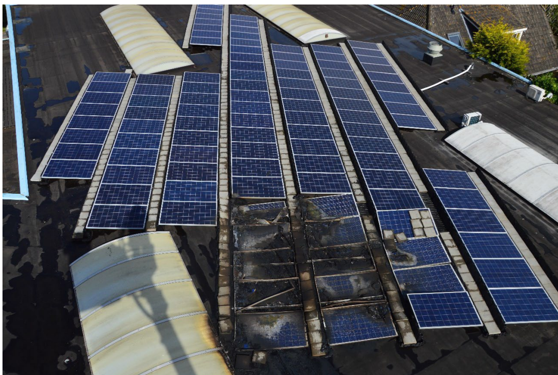
Figure 13 Damage on the roof (source: TBO Fire Department Haaglanden)
