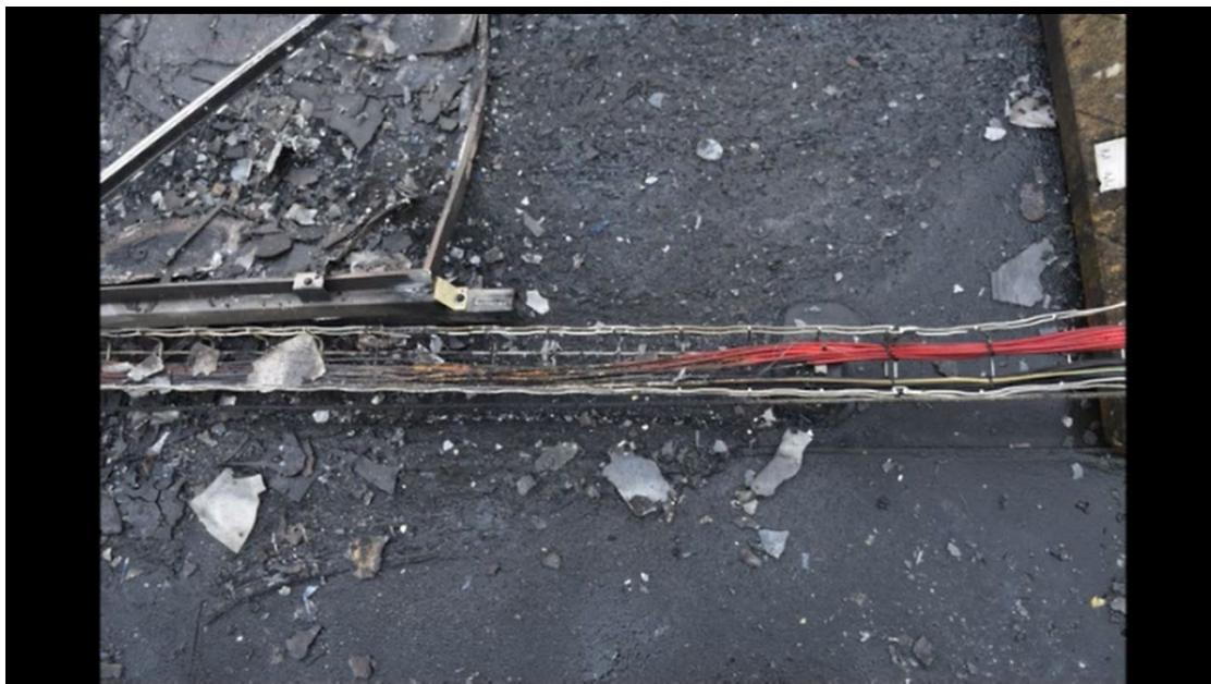
Figure 18 Damage to the cables (Source: Gelderland-Midden Fire Brigade)
